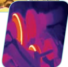
Pulley System: Hot Drive Belts
